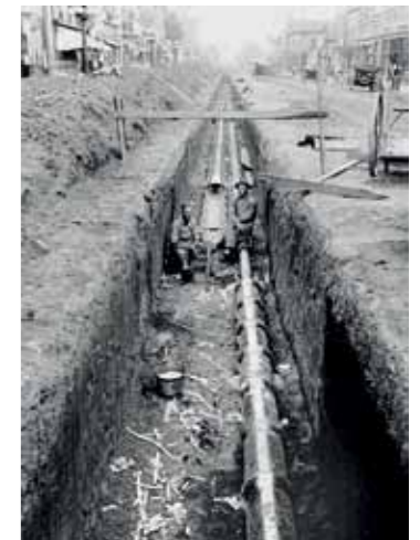
Figure 3. Pipe laying in 1880, unencumbered by a proliferation of other buried utility services, and health and safety legislation. Courtesy of www.sewerhistory.org
